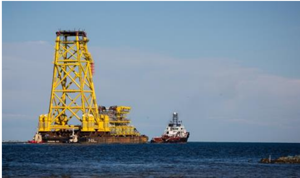
Figure B-4 Tyra SE-B facilities (jackets, top side and bridge) – tugged to location in 2014
