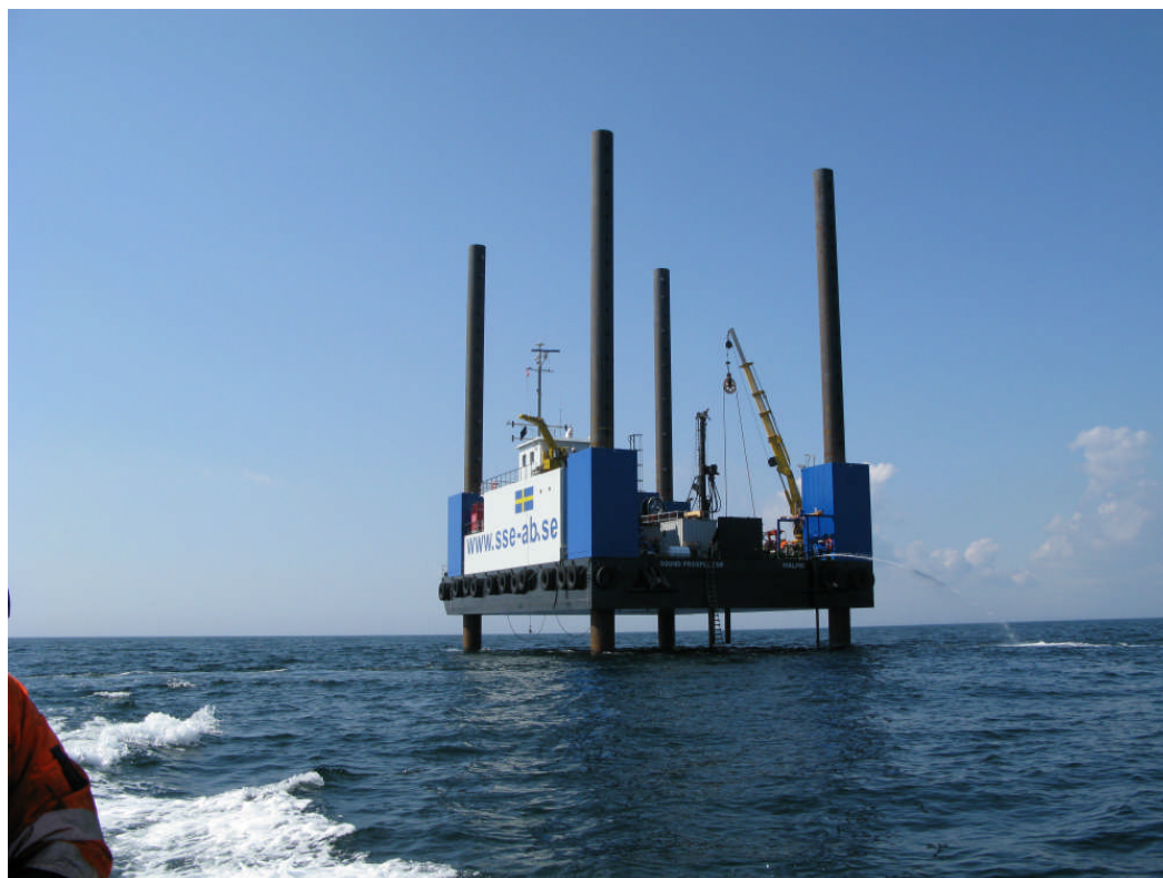
Picture 2.1: Sound Prospector equipped with GEOs drilling rig on the Anholt Offshore Wind Farm project
