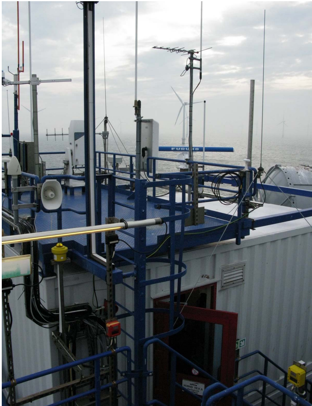
Technical installations including radar at Horns Rev 2 © Thomas W. Johansen
