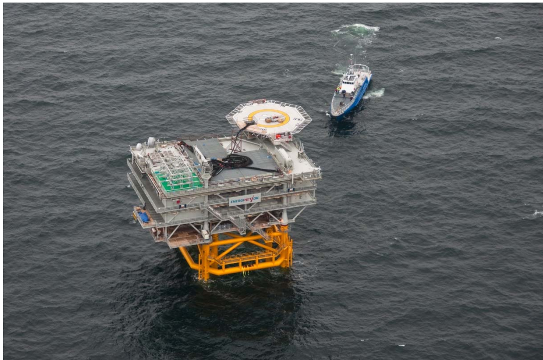
Transformer platform and crew boat – Anholt Offshore Wind Farm
