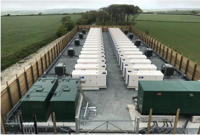
Figure 2 Emergency plant in Cornwall. Photograph: SEA Trasformatori
