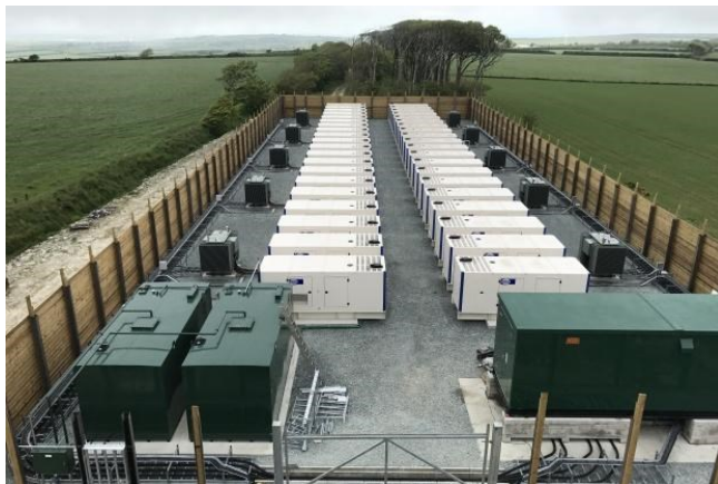
Figure 2 Emergency plant in Cornwall. Photograph: SEA Trasformatori
