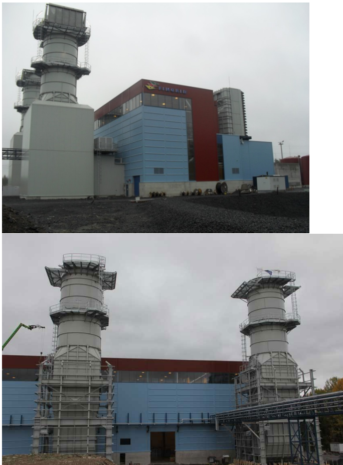
Figure 3 Forssa Power plant commissioned for Fingrid [17].
