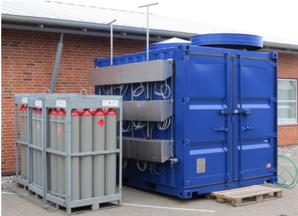
Figure 2: A 50 kW LT-PEMFC CHP hydrogen unit from Dantherm Power.
