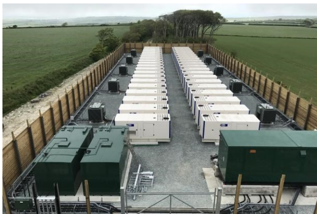
Figure 2 Emergency plant in Cornwall. Photograph: SEA Trasformatori
