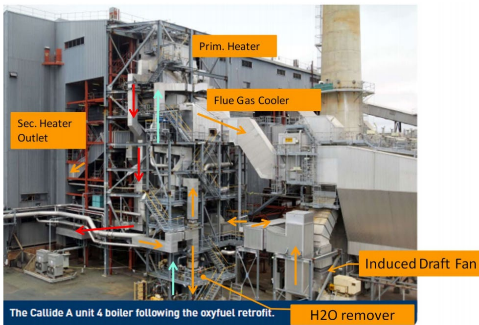
Figure 0-10 Photo of Callide Oxy-fuel boiler from [52] showing retrofit paths (red) and flue gas flow directions (yellow).
