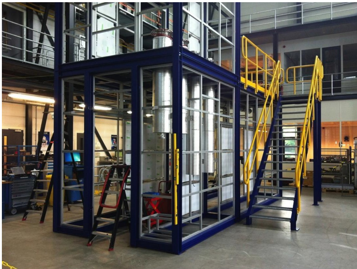
Figure 4 Haldor Topsøe SNG Pilot Plant
