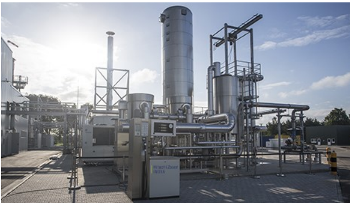
Figure 3 SNG Methanation Plant
