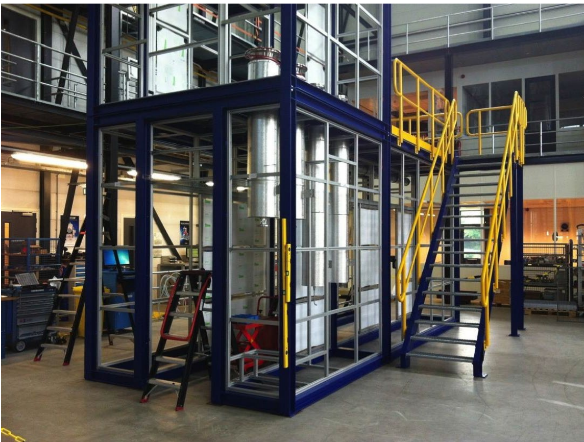
Figure 4 Haldor Topsøe SNG Pilot Plant
