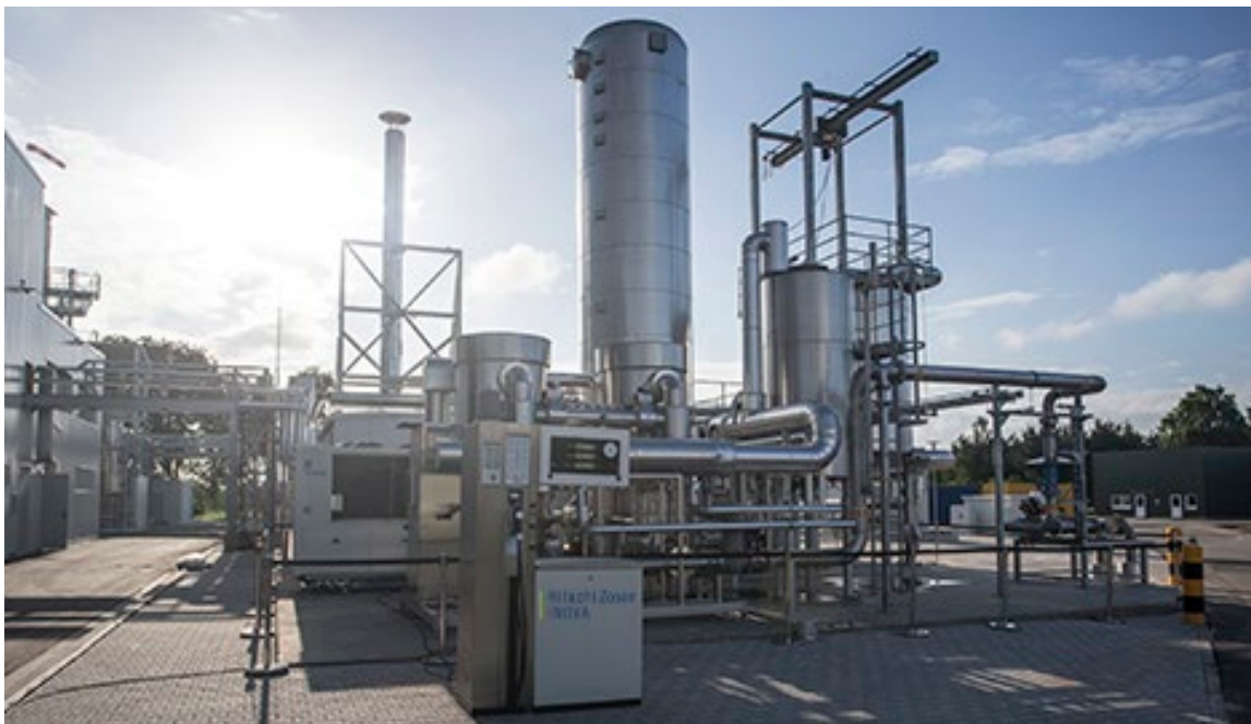
Figure 3 SNG Methanation Plant
