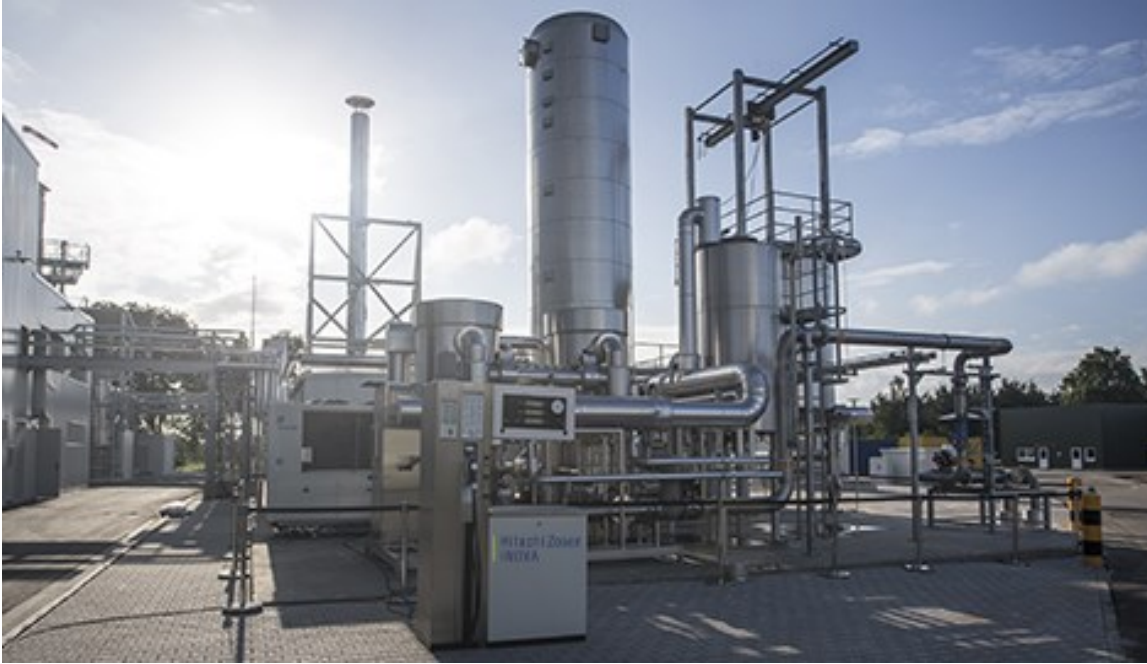
Figure 3 SNG Methanation Plant
