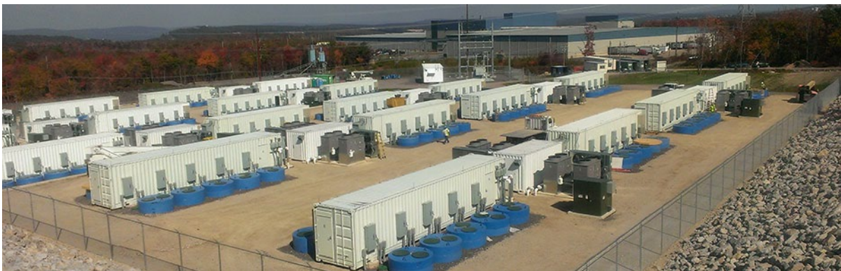
Figure 5: Photo of Beacon Power flywheel installation in commercial operation in PJM, Hazle, Pennsylvania. The plant includes 200 flywheel modules lowered into the ground (5 on each side of a container). The plant currently provides 20 MW of frequency regulation service to PJM and reached full commercial operation in July 2014 [6].
