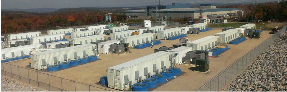
Figure 5: Photo of Beacon Power flywheel installation in commercial operation in PJM, Hazle, Pennsylvania. The plant includes 200 flywheel modules lowered into the ground (5 on each side of a container). The plant currently provides 20 MW of frequency regulation service to PJM and reached full commercial operation in July 2014 [6].
