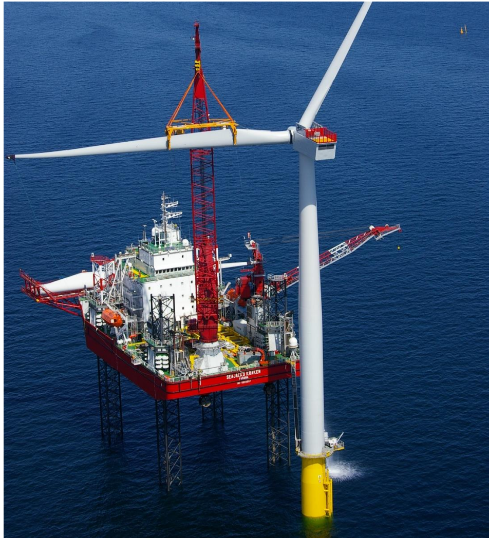
Figure 2.2: Turbine installation using a jack-up vessel. The illustration is not necessarily applicable to the current project where different solutions for foundation structures are included.
