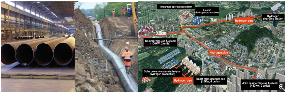
Figure 30: Equipment, installation and difficulties associated with installation in larger cities
