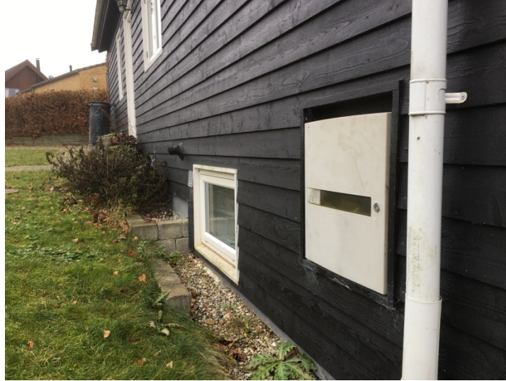
Figure 4 Cupboard containing pressure regulator and flowmeter mounted outside a private house.
