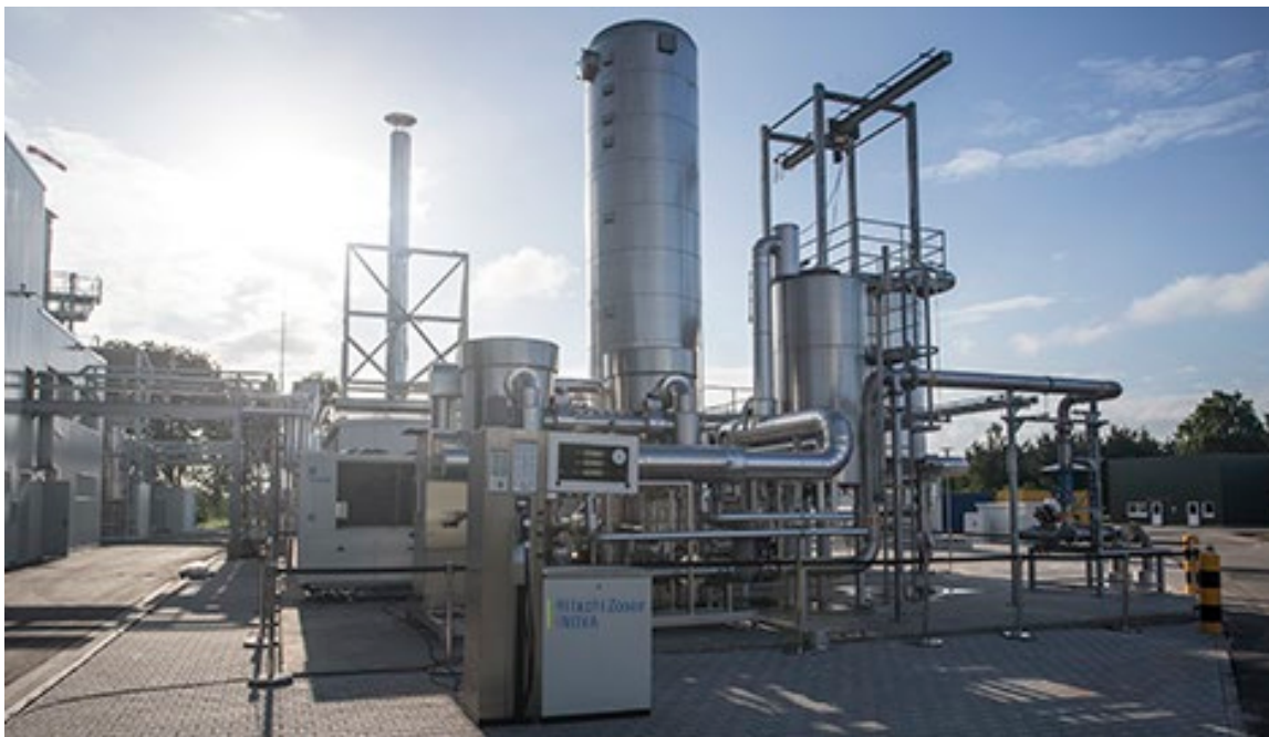
Figure 3 SNG Methanation Plant
