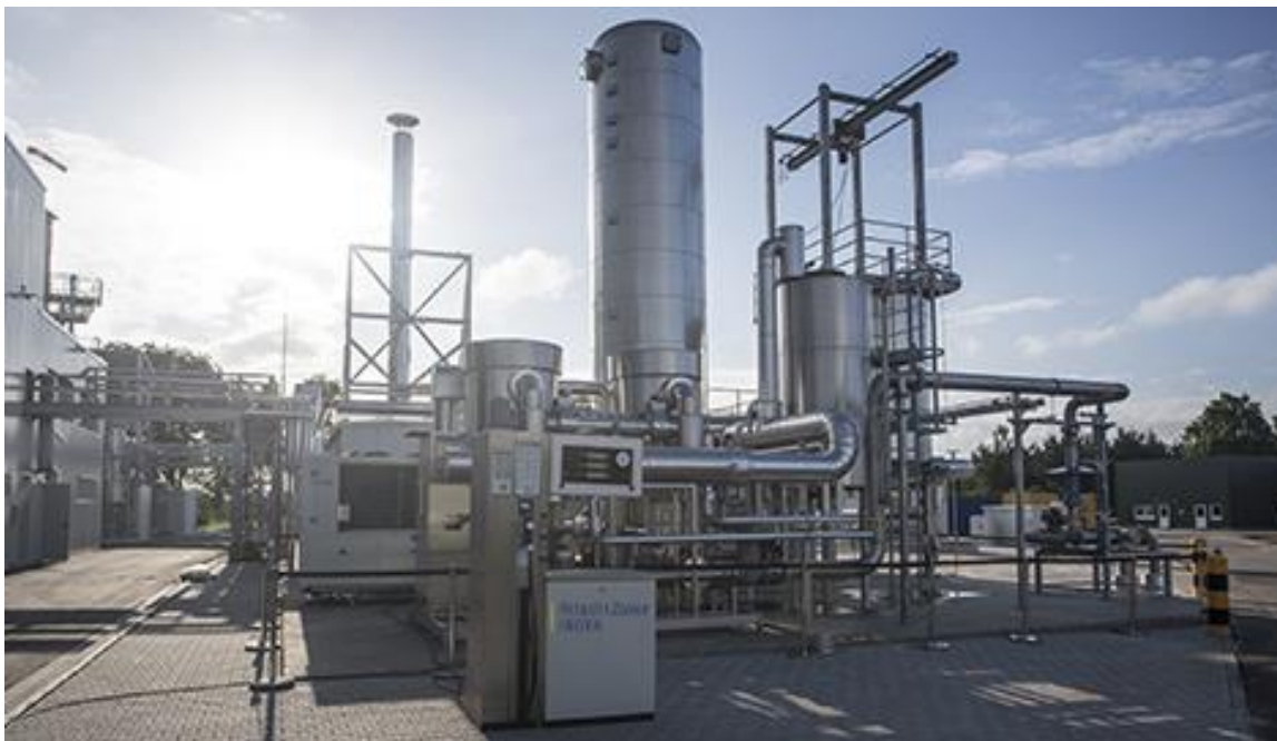
Figure 3 SNG Methanation Plant
