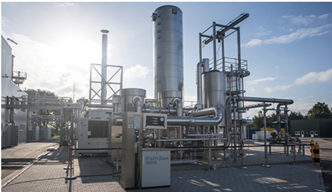
Figure 3 SNG Methanation Plant
