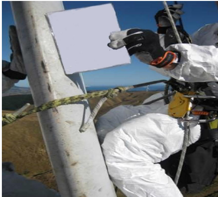
Figure 1. Example of observed leading edge erosion in the field.
