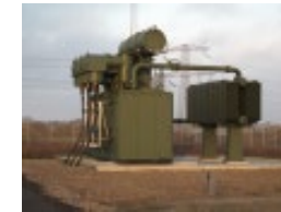
220 kV shunt reactor
