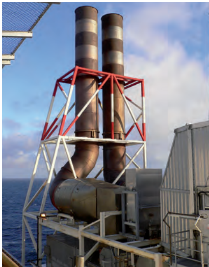
Exhausts from gas turbines on the South Arne offshore installation.
