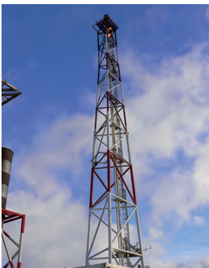
Flare stack on the South Arne offshore installation.
