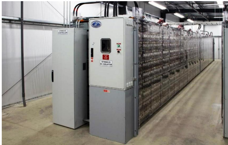
Figure 2.26. Three strings of batteries installed. Source: (DOE, 2015)
