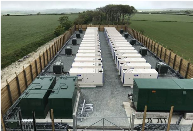
Figure 2 Emergency plant in Cornwall. Photograph: SEA Trasformatori
