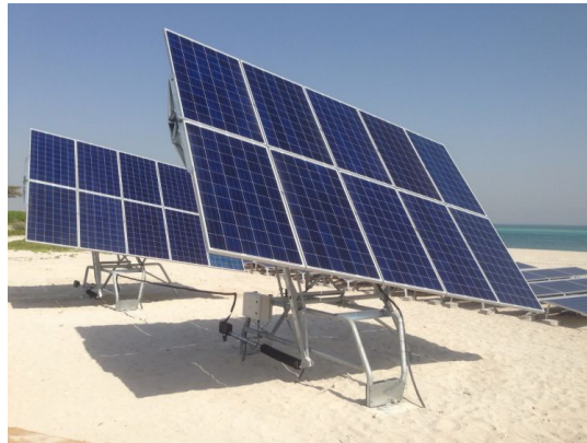
Figure 6 A Helioslite 1.5 tracking system (Ref. 13).
