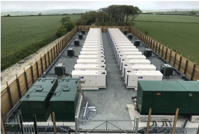
Figure 2 Emergency plant in Cornwall. Photograph: SEA Trasformatori
