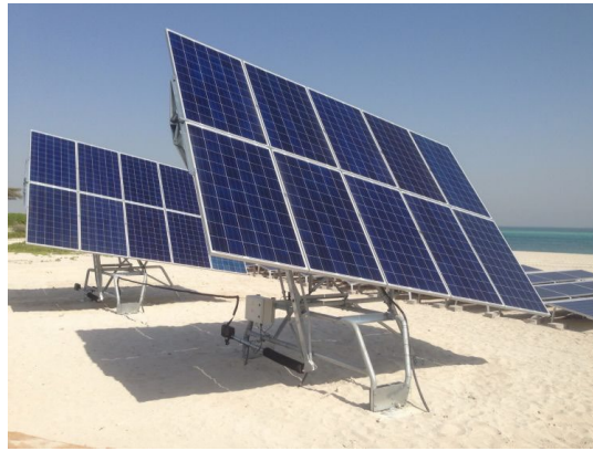
Figure 6 A Helioslite 1.5 tracking system (Ref. 13).
