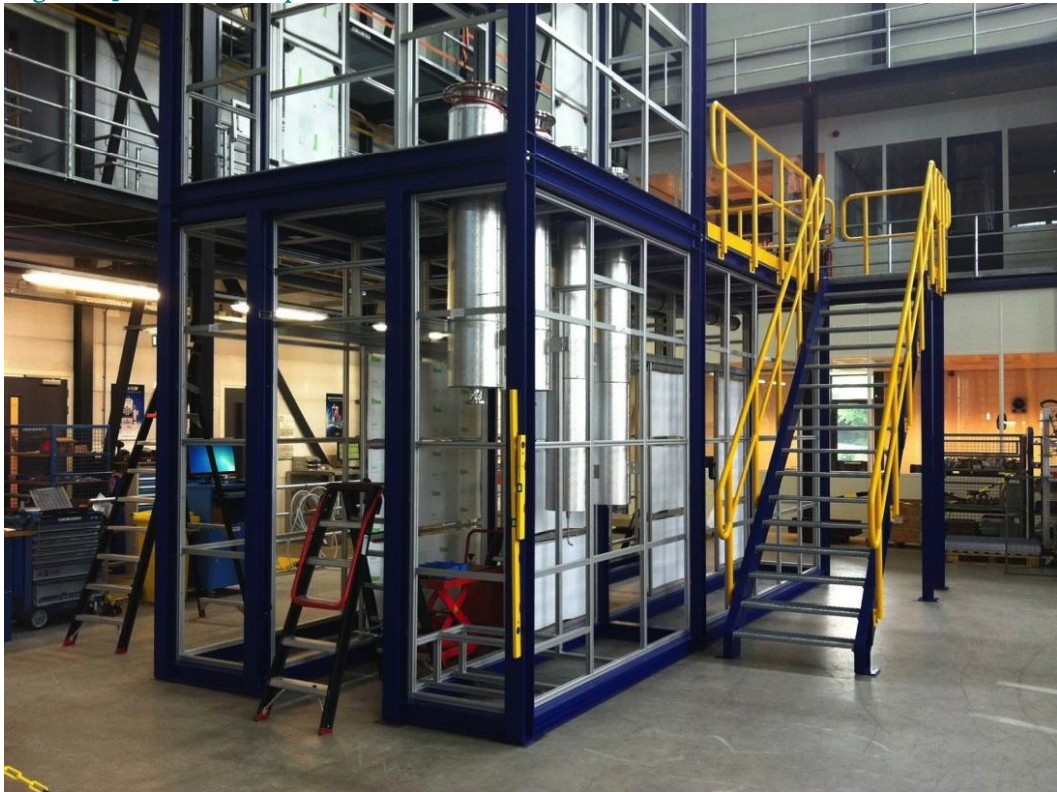
Figure 4: Haldor Topsøe Methanation Pilot Plant
