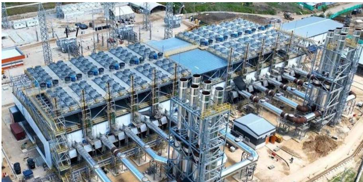
Figure 91. El Tesorito Power Plant, Sahagún, Colombia [11].
