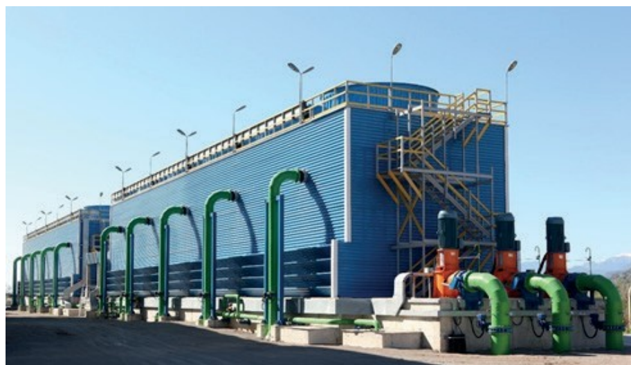
Figure 15: Industrial cooling towers for a power plant
