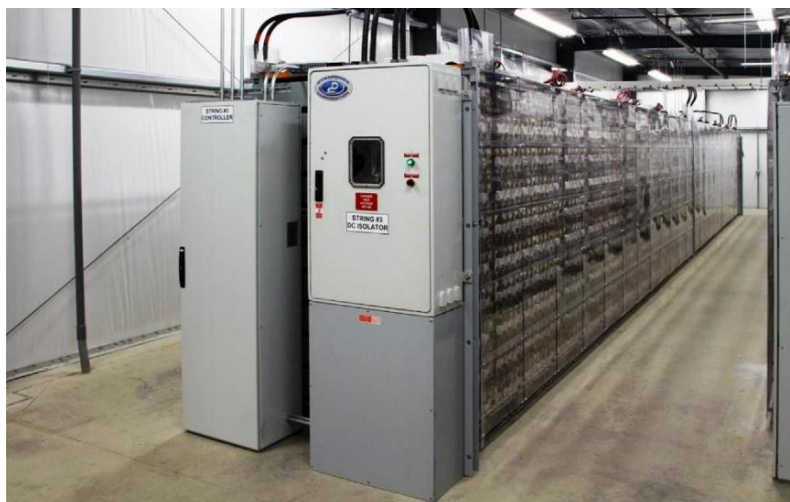
Figure 2.26. Three strings of batteries installed. Source: (DOE, 2015)
