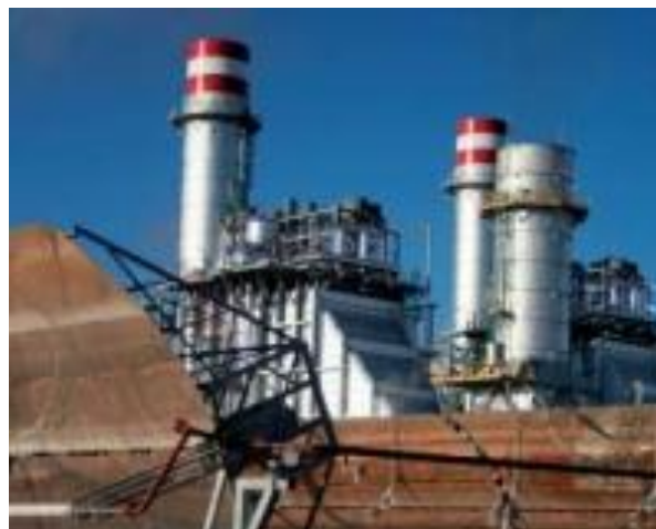
Figure 2.46. Ain Beni Mathar power plant. Source: (ABENGOA, 2019)
