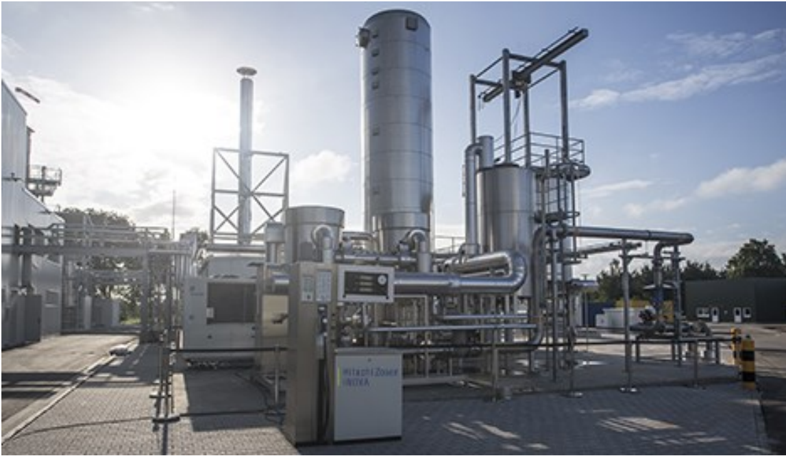
Figure 3 SNG Methanation Plant
