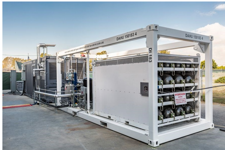
Figure 2: SOEC hydrogen plant from Sunfire [11].
