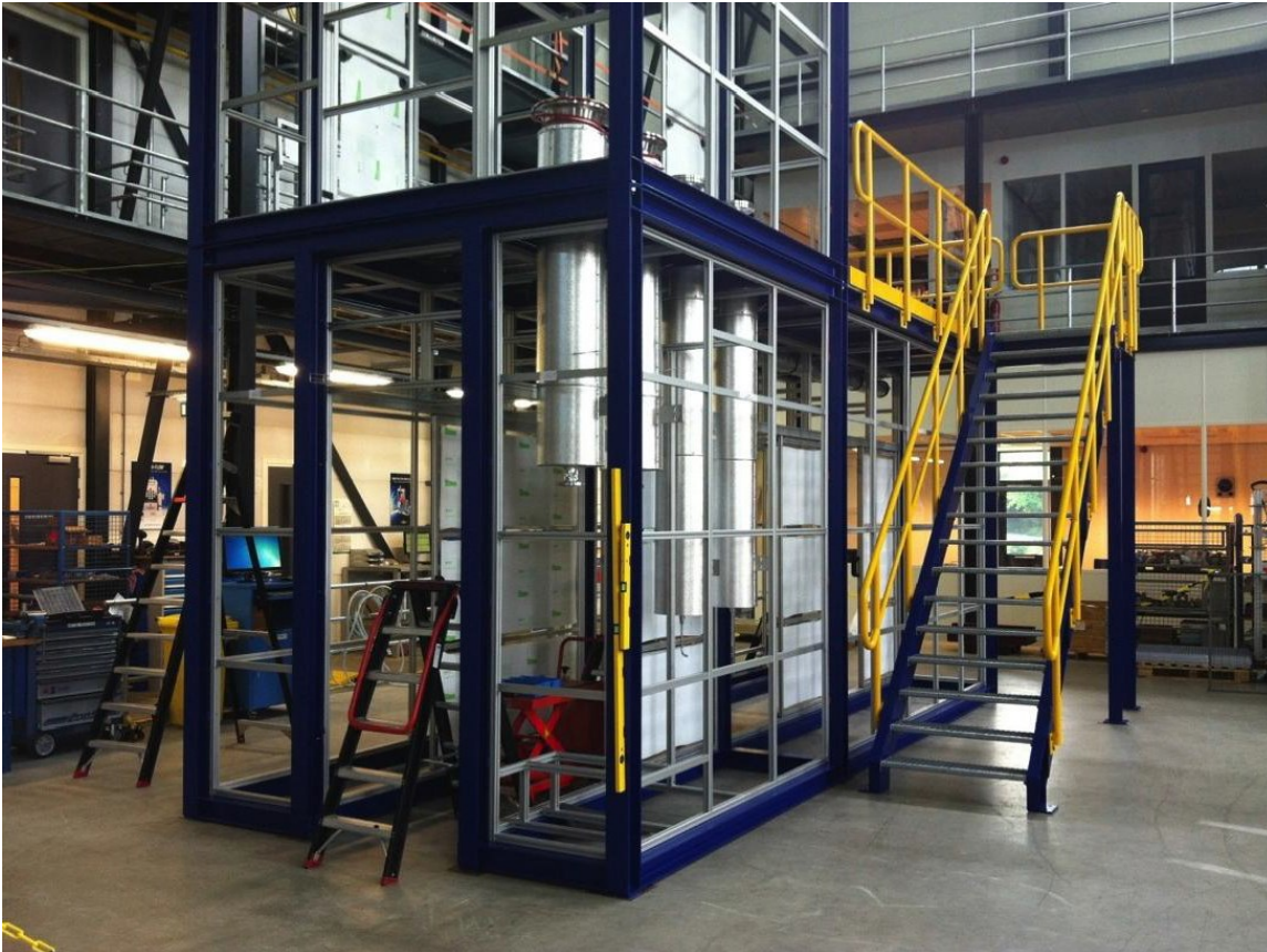
Figure 4 Haldor Topsøe SNG Pilot Plant
