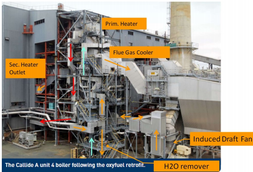
Figure 31 Photo of Callide Oxy-fuel boiler from [11] showing retrofit paths (red) and flue gas flow directions (yellow).
