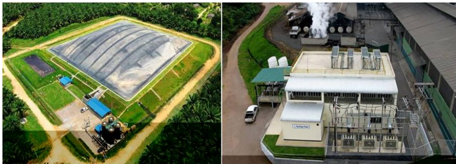
Covered lagoon type – biogas power plant of PT REA Kaltim Plantations (ref. 10)
