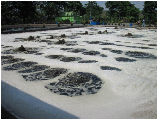
Leachate collection and treatment pond at Bantar Gebang Landfill gas power plant. (ref. 8)
