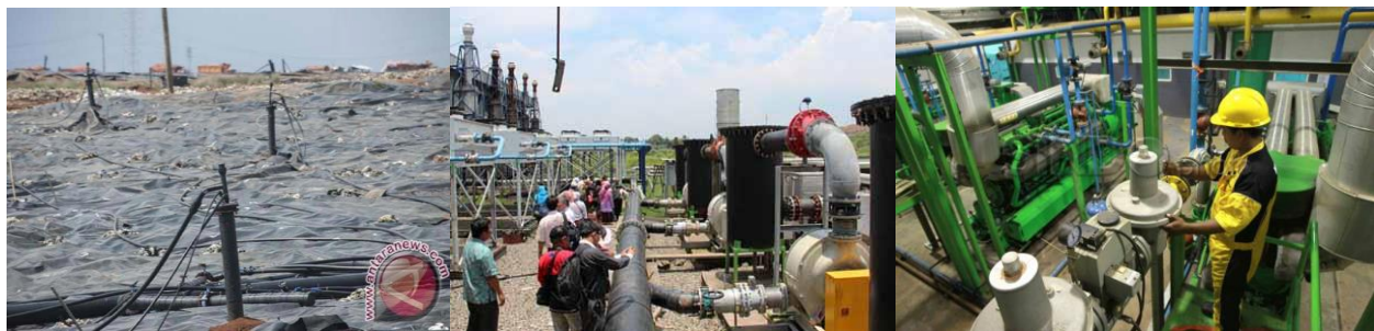
Land-fill gas power plant at Bantar Gebang, Bekasi, West Jawa (ref. 13)
