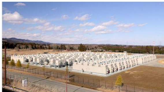
Picture of the 40 MW and 40 MWh energy storage system in Fukushima, Japan.
