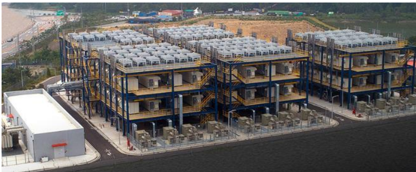
50 MW byproduct-hydrogen-fuel-cell power plant located in Seosan, South Korea. (Ref 10)
