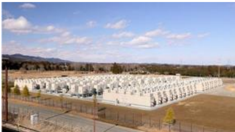
The 40 MW and 40 MWh energy storage system in Fukushima, Japan.
