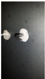
Pressure tap, not in flush with internal casing
