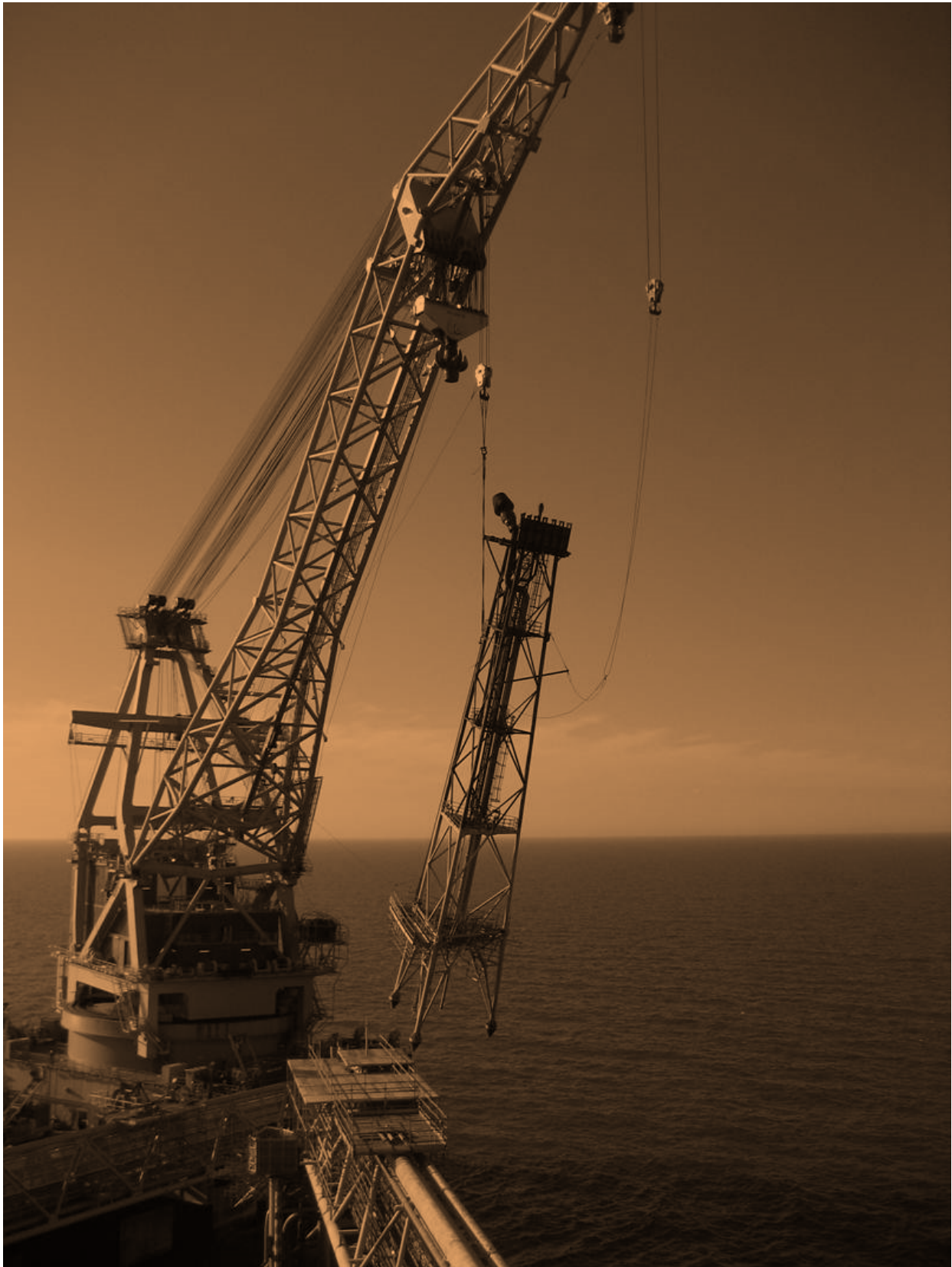
Replacement of flare tower on the Tyra West platform. Foto: Stig Busk Jespersen
